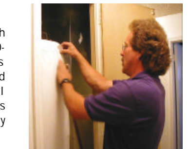
Michael Guella is shown wrapping Karen's hot water heater; the heating vent system will be rechecked before the crew leaves the job site.
