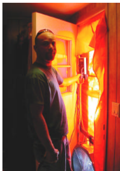
Warnell Jones, a contractor for CSA in Reno, installs a blower door to test air infiltration.
